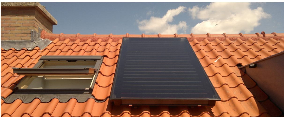
Solar system installed on the roofs of buildings in the Delft pilot site
