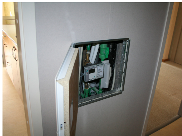
Meter for DHW in one apartment
