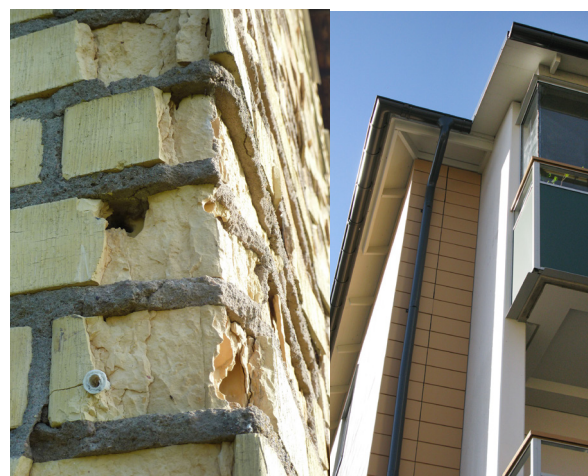
Crumbling brick façade before and the new tile facade after the refurbishment.
