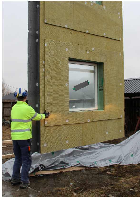
A sample of the new mock-up wall, which is prefabricated and transported to the construction site
