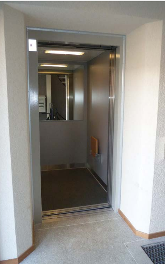
Newly installed lift
