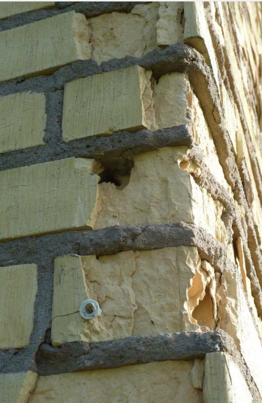
Bricks affected by frost wedging
