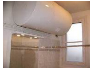
Fig. 7 Individual electric boilers in bathrooms
