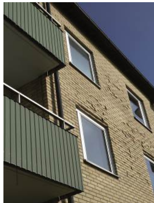
Fig. 12 Technical flaws at Brogården - thermal bridges by indented balconies and crumbling bricks on the facade
