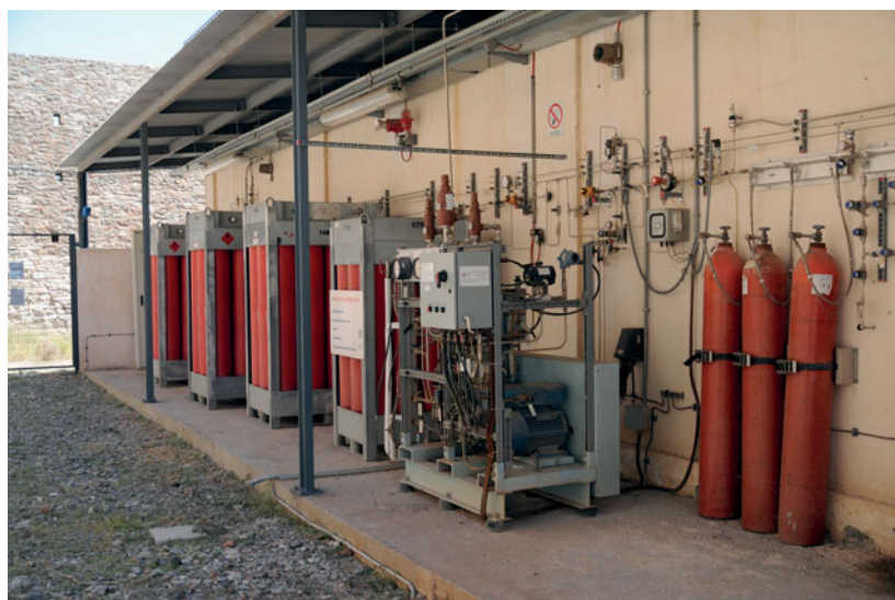
Hydrogen storage and distribution grid
